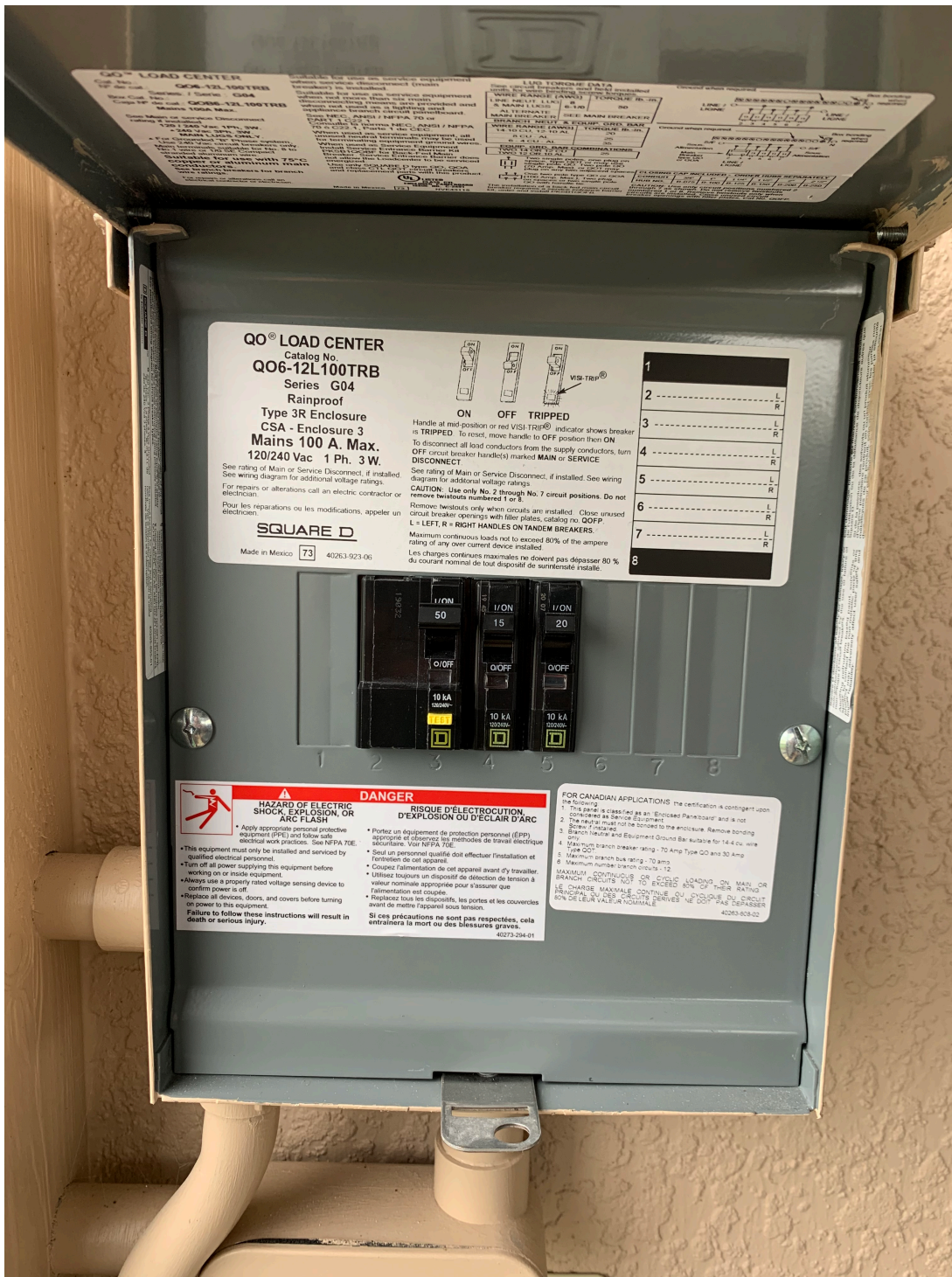
My current electrical service with additional capacity.
