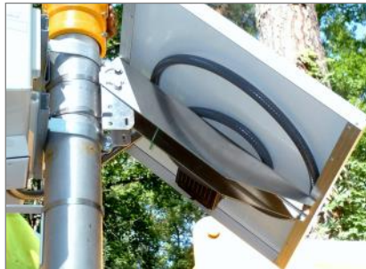
50-watt solar panel bracket mounted on pole
